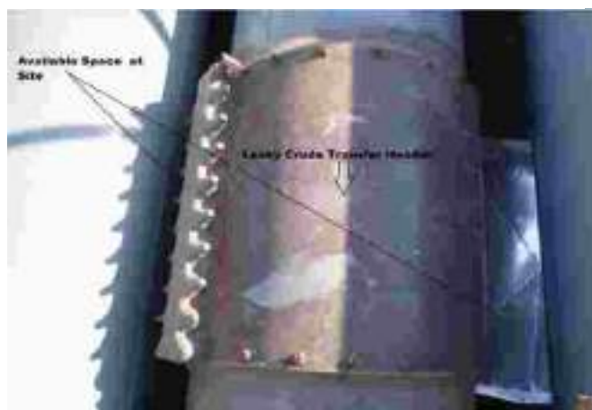
Figure I-3.2: Example of temporary safety measure to prevent new contamination from spill. The clamp is applied to stop a leak on a leaky pipe header running
